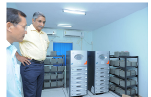
Secretary(Power) & MD, GUVNL at battery room of CCC
