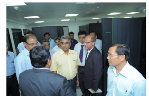
Secretary (Power) & JS discussing about data center with TCS officials
